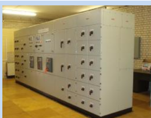
The New LVAC Board All Circuits were migrated to this board without ever requiring the sub-station to leave service.
