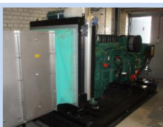
And for the Next 40 Years... The new WARDPOWER WP-V377PXD Diesel Generating Set designed with a 40 year asset life.
